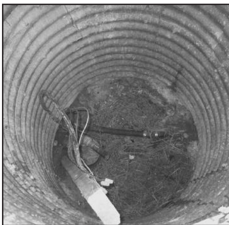
Drilled well in a pit.
