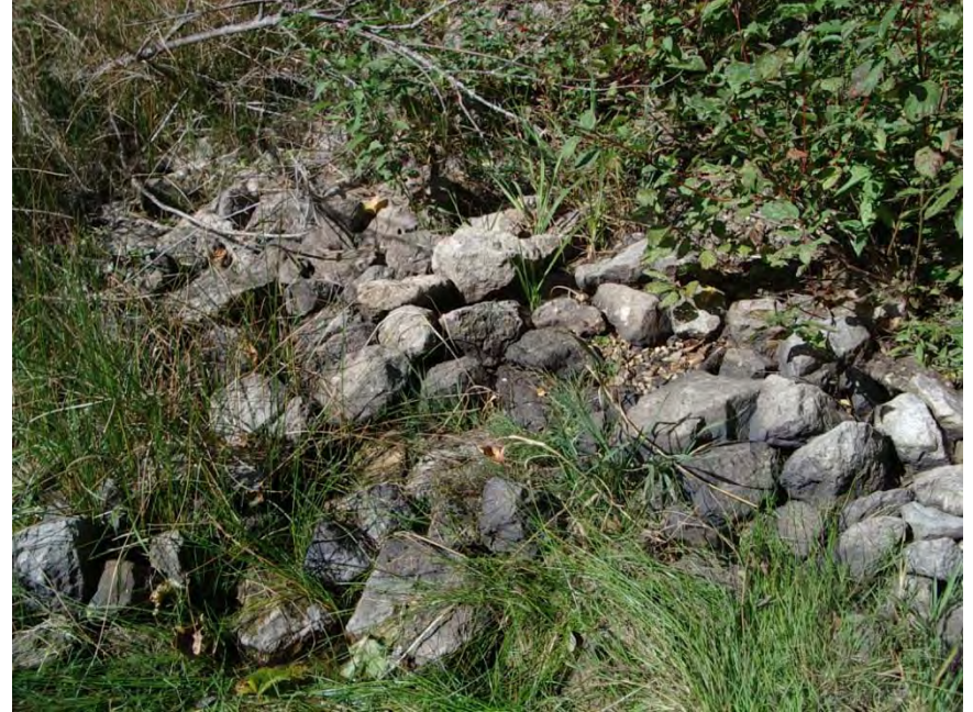
Photo 28 – View showing Wetland W7 Diffuse Discharge Inflow. Note that the gabion stone used to armour the diffuse discharge is now well-worn, 7 years after it was installed. GEC 2017-10-01
