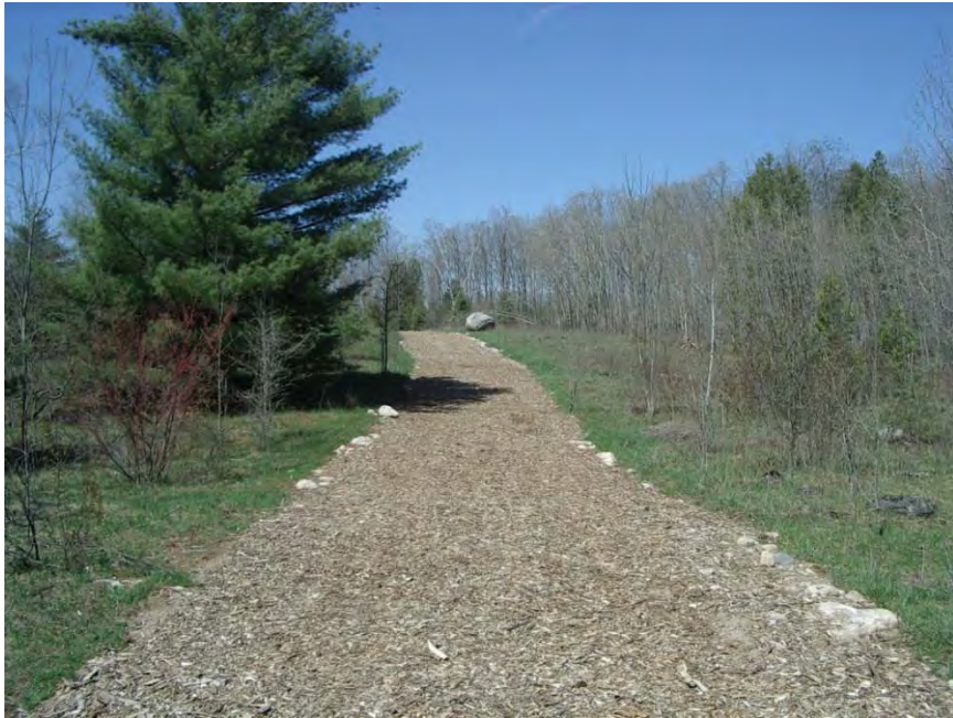
Photo 9 - View showing recently buried feeder lines leading to Recharge Wells RW203C, RW203D, RW204C and RW204D, with a 15-20 cm deep layer of fresh wood chips. GEC - 2013-05-04
