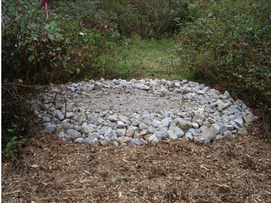
Photo 23 – View of Wetland W7 Diffuse Discharge Inflow, shortly after installation in 2010. GEC 2010-09-30
