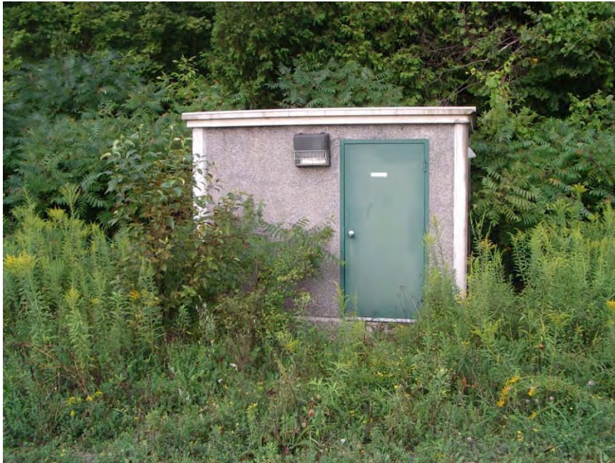
Photo 5 – View of a typical Control Valve (CV) Hut. Vegetation becomes re-established around the huts relatively quickly. GEC 2018-08-26
